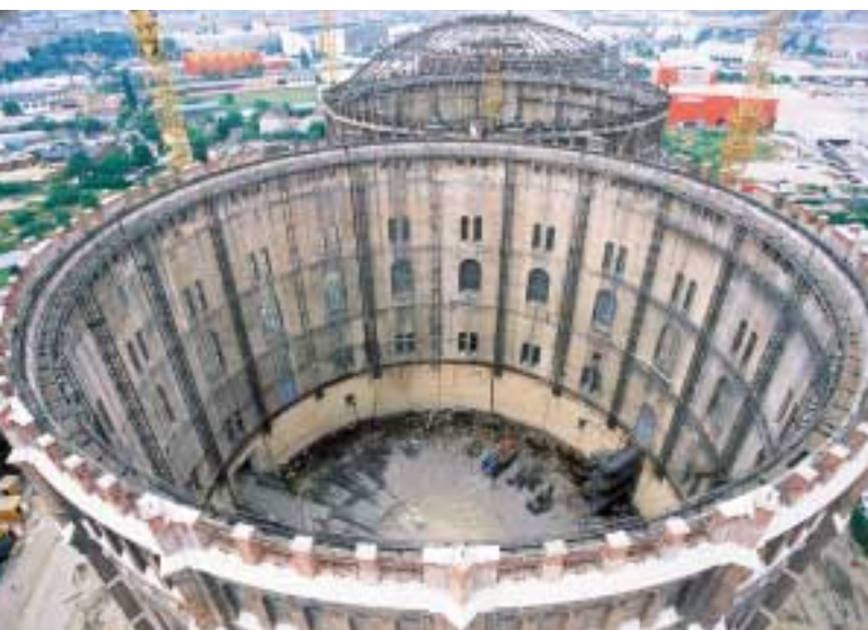
Photo far left: Stefan Götz measures the dome structure with the LEICA TCRA1105 in automatic reflectorless sensor ranging mode. Left: Gasometer C and D at different stages of renovation. Photo: Porr/Rappersberger
