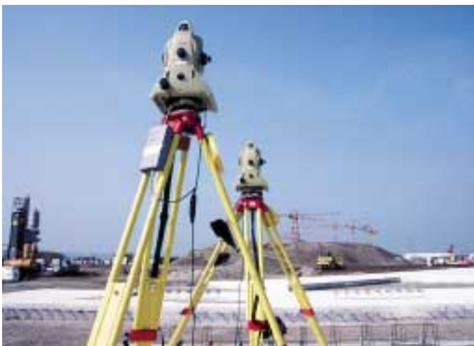
Two LEICA TCA2003 total stations track the slip-former position in real time.
