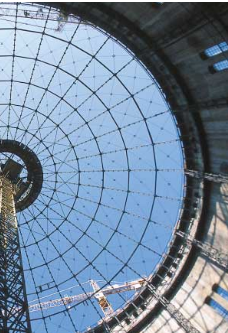
Left: The 160 ton steel dome structures were renovated. With a central scaffolding the pressure ring was placed underneath. Photo: Porr/Gruna
