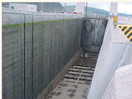
Cracks at the end of this concrete structure were scanned for assessment purposes. Image courtesy: David Evans and Associates
