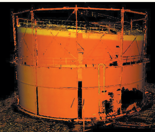
This collapsed 100' diameter tank was scanned to assess whether it could be saved or should be demolished. Image courtesy: North Surveys
