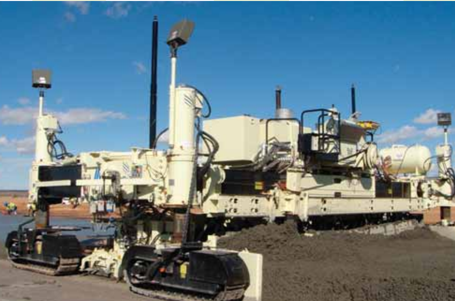
Two prisms, attached to each side of the Guntert & Zimmerman S850 paver, receive signals from the two robotic total stations set up on tripods ahead of the paver.
