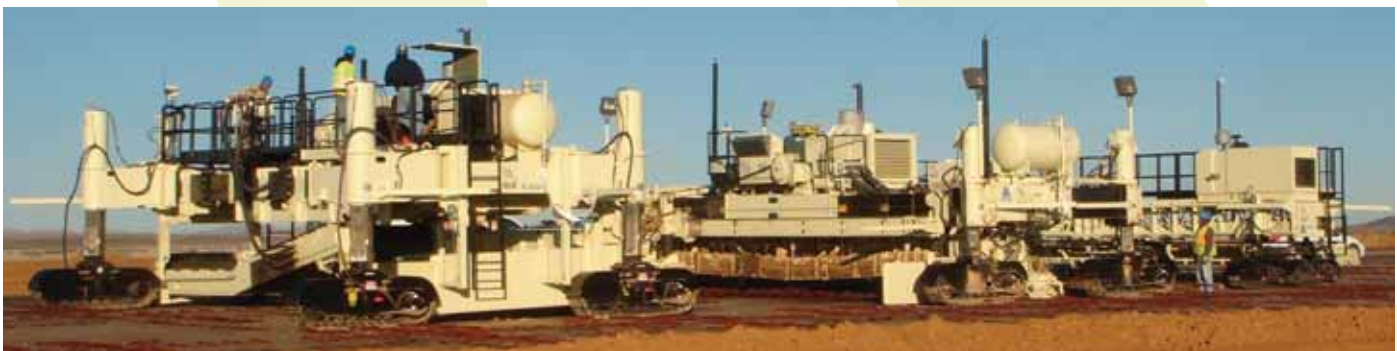
The all-new paving spread for Spaceport America consists of a placer-spreader, at left, followed by the paver and a texture-cure machine.
