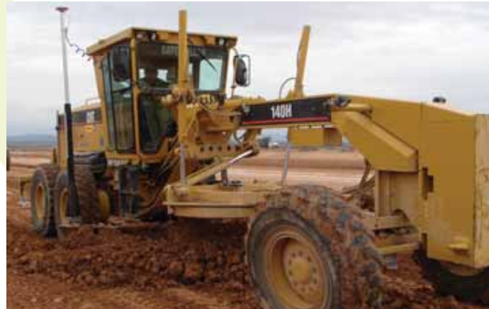
A Leica PowerGrade 3D GPS system controls a Caterpillar 140H motor grader. The system doubled production on the 10,000-foot runway at Spaceport America in New Mexico.
